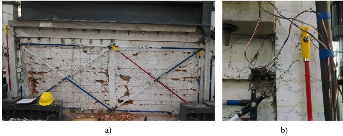
Fig. 11. Crack pattern of specimen MD3NRH. (a) Cracking on the wall, (b) beam-column connection failure.
