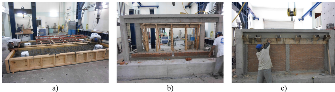
Fig. 5. Construction stages of the specimens. (a) Foundation construction, (b) Specimen construction, (c) Casting of upper tie beam.
