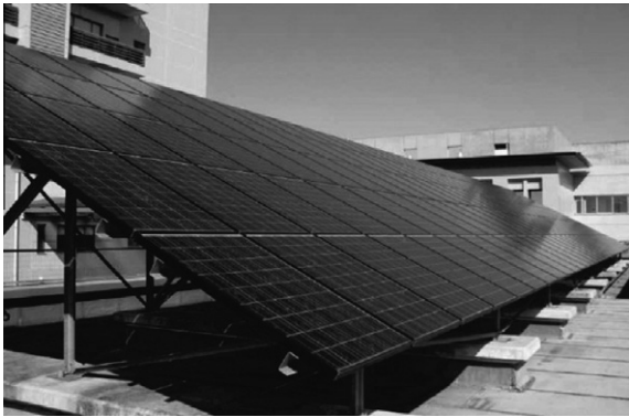
Fig. 2. The studied photovoltaic field installed at Tokyo University of Agriculture and Technology.
