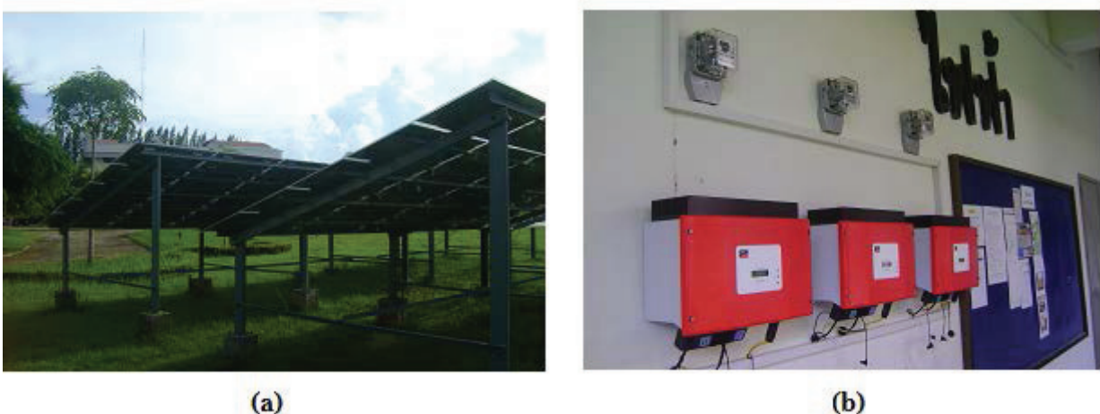
Fig. 3 shows the solar plant real location (a) and the inverter for connect the electrical power system (b).
