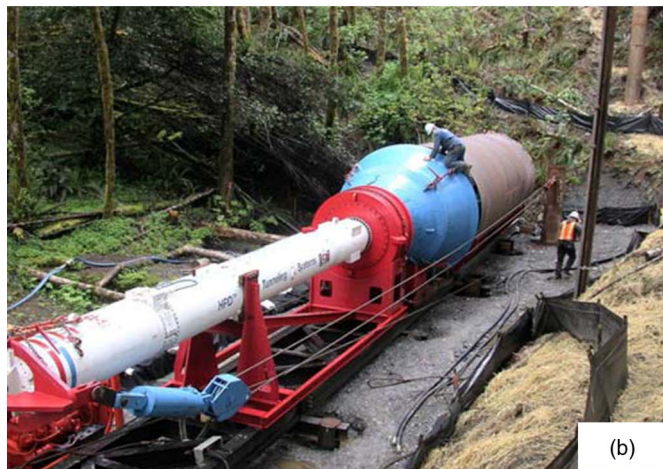
Fig. 2. (a) 610 mm pneumatic hammer driving 1,070 mm diameter pipe; (b) hydraulic hammer driving 3,050 mm diameter pipe (adapted from Piehl 2005)
